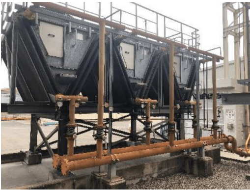
10. The existing lube oil fin fan cooler is undersized so a new one is needed. Courtesy: Siemens Energy
