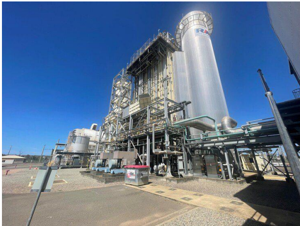
2. The Townsville Power Station in Queensland, Australia. Courtesy: Siemens Energy
