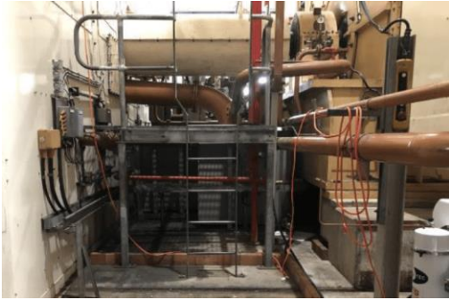
9. The existing lube oil tank is directly under the intermediate shaft. A new tank with enclosure needs to be installed outside the turbine hall. Courtesy: Siemens Energy
