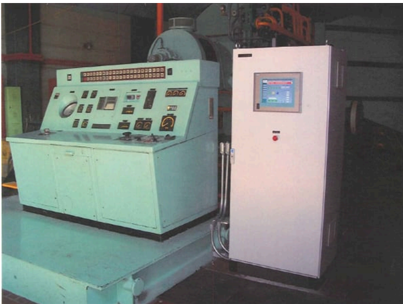
7. Upgraded controls. The 1970s-vintage analog controls (left) were upgraded with a digital control system (right) that managed the new sequencing and control requirements of the plant. The combustion turbine startup sequencing management remains with the original controls. Courtesy: Industria Sigrama
